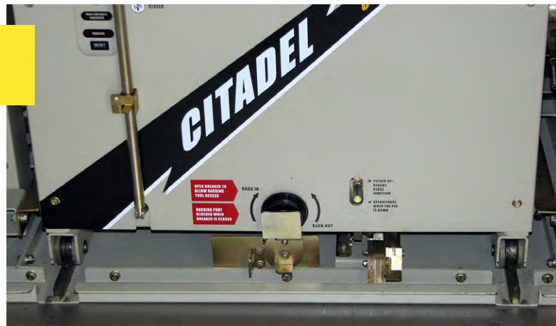
Locked in disconnect position
