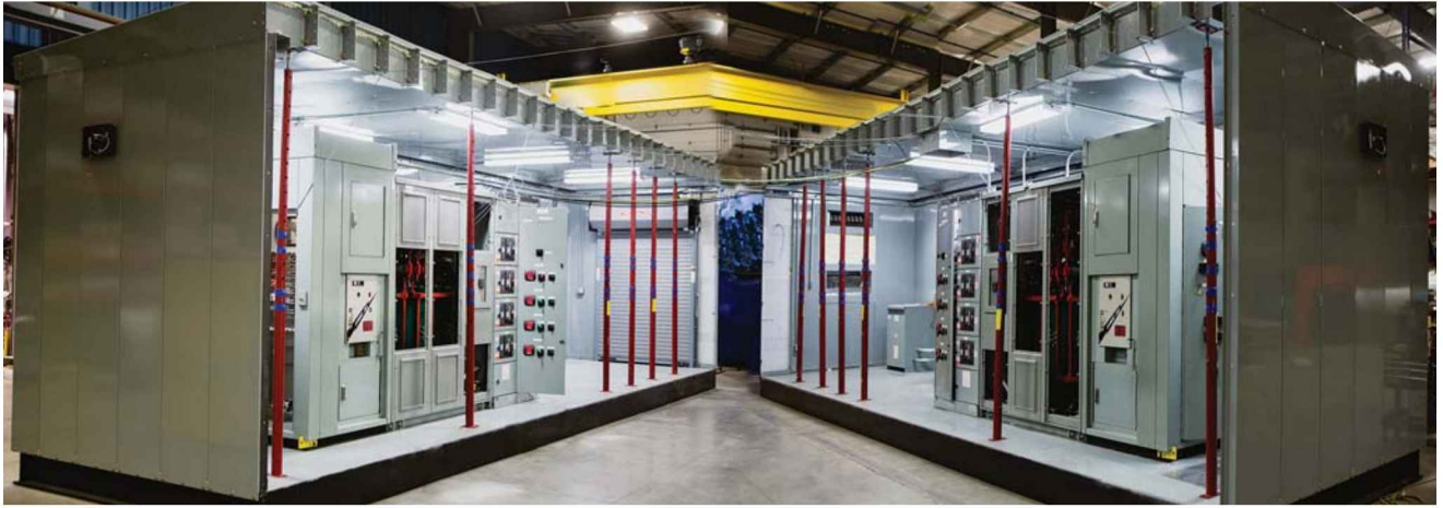
If the water treatment goes down, the plant goes down. Unit substation has 100% mirror image redundancy.
