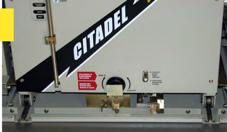
Locked in disconnect position
