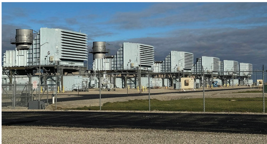
1. Generating plant features multiple 7EA simple-cycle peakers
