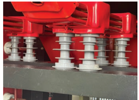
8. With Crown-sulators in place, switch-gear has better mechanical bracing and dewpoint-rated hi-pot withstand
